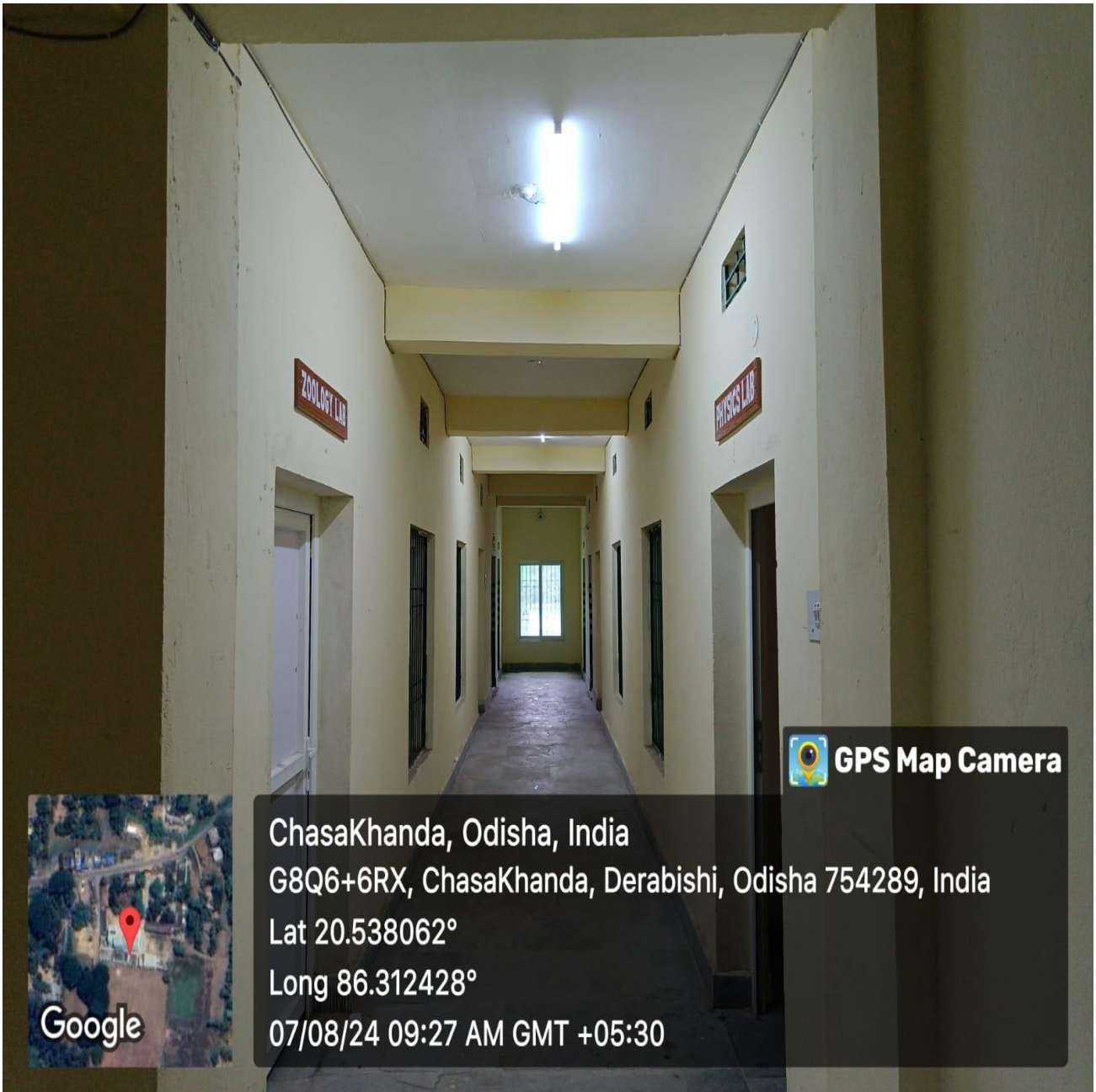
Led Lights in Building Corridors
