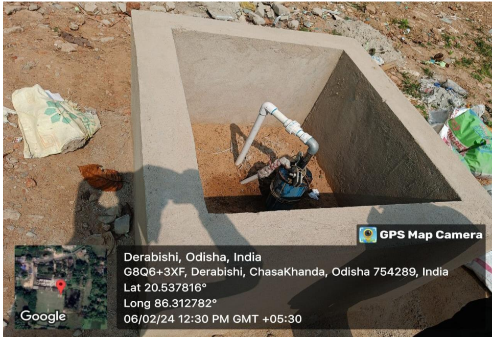
(Photograph of Overhead tank which supplies water to the institute)
