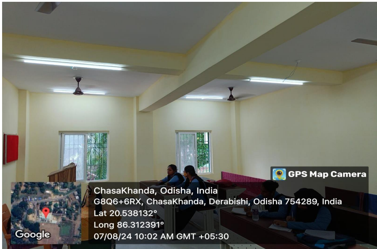
LED Lights in Class Room
