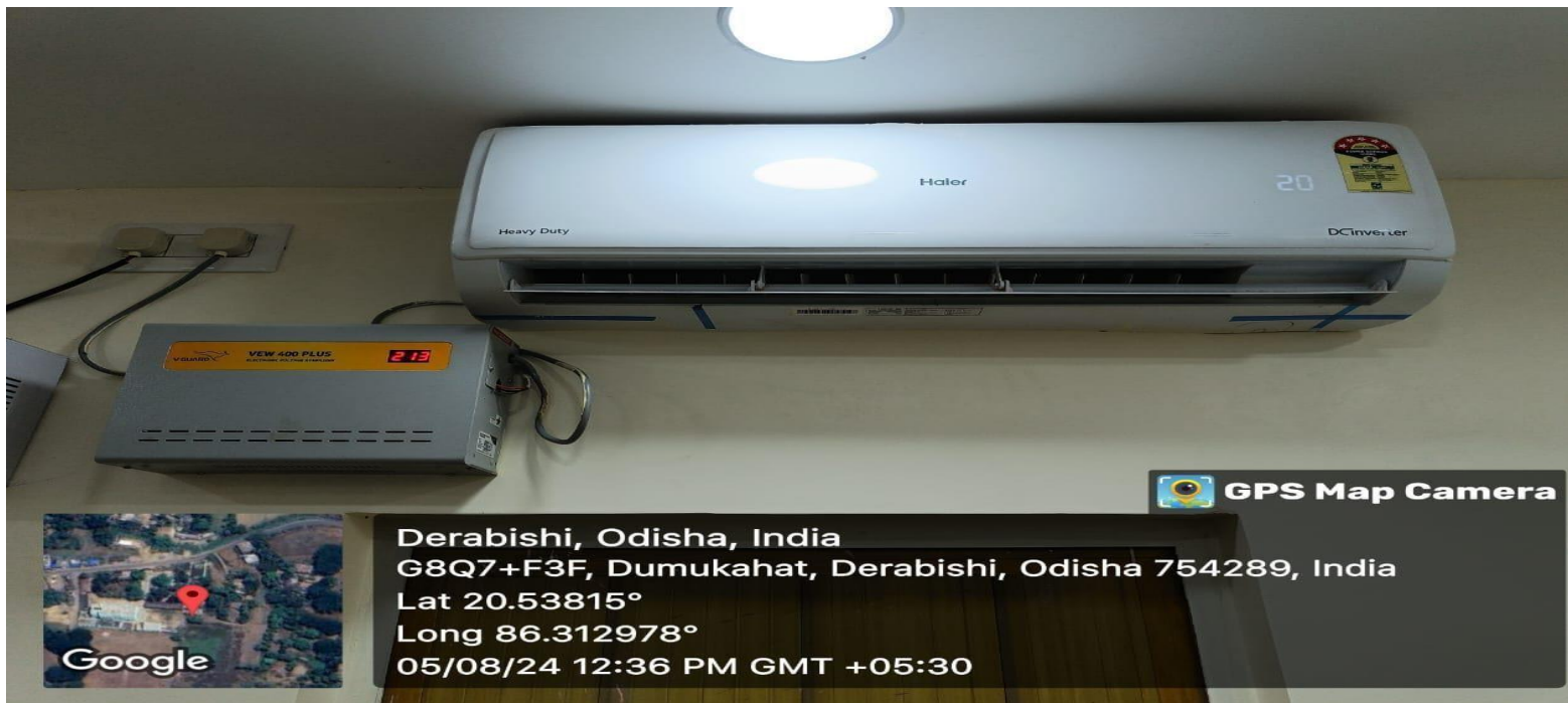
(Energy efficient Air-Conditioner)
