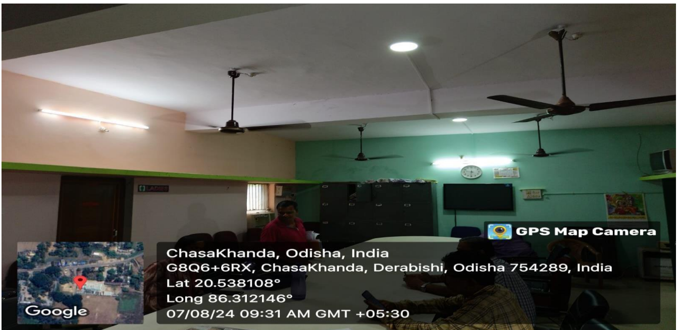
LED Lights in Staff Common Room
